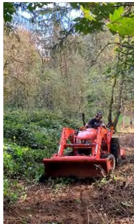
NR Technician, AJ Ulibarri brush hogging in preparation for new fence installation
