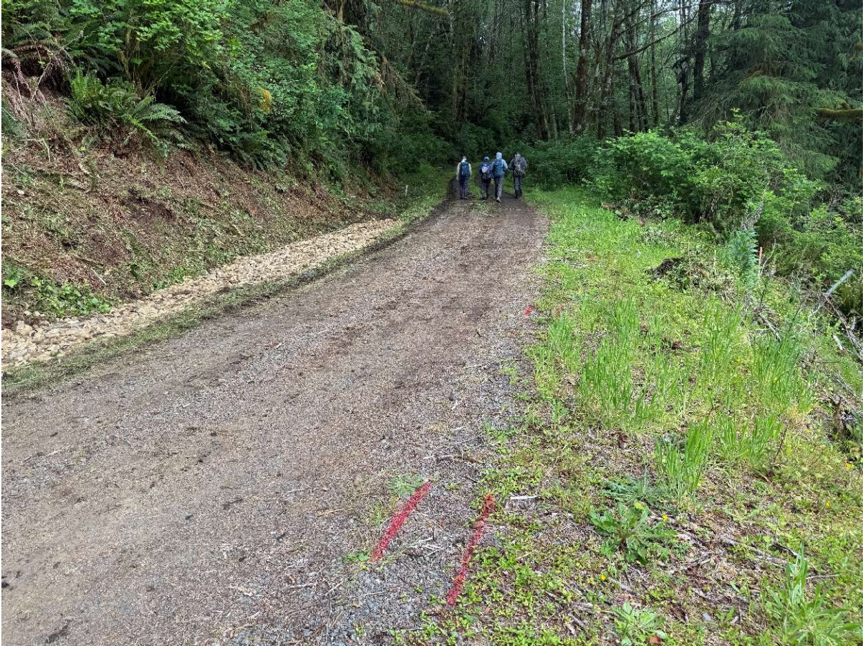
9. Photo near what WDFW refers to as the “riverside slide” area. WDFW recently placed additional rock. Photo from 5/20/2026.
