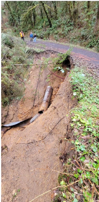
Photograph 1: Original Slope Failure
