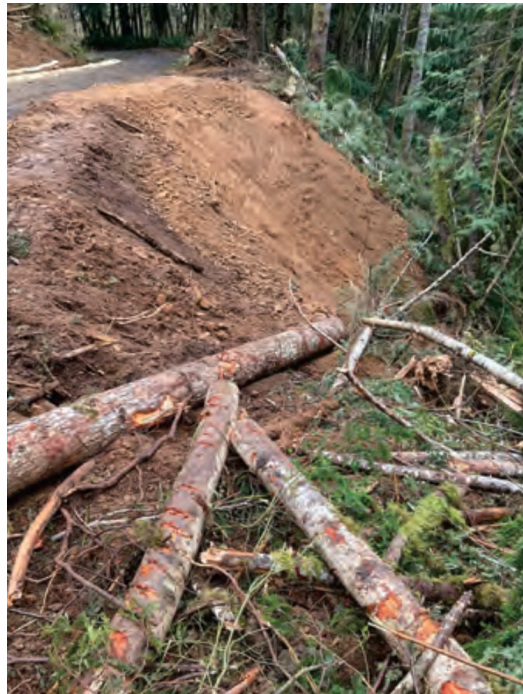
Photograph 2: Backfilled Original Slope Failure
