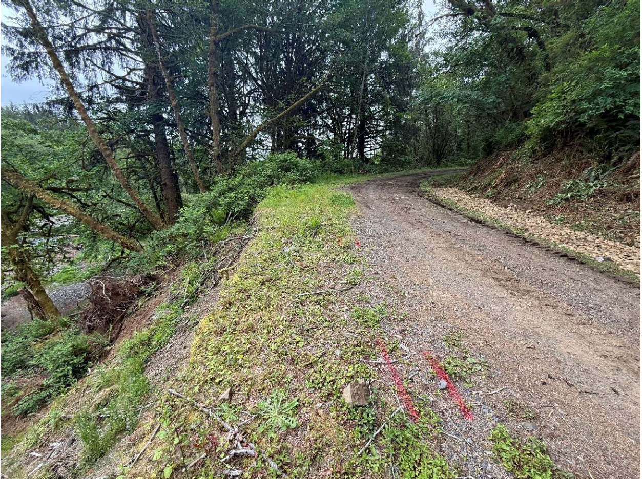
7. Photo near what WDFW refers to as the “riverside slide” area. WDFW recently placed additional rock. Photo from 5/20/2026.
