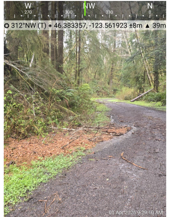
Photograph 3: Choked Ditch with Runoff now in Roadway
